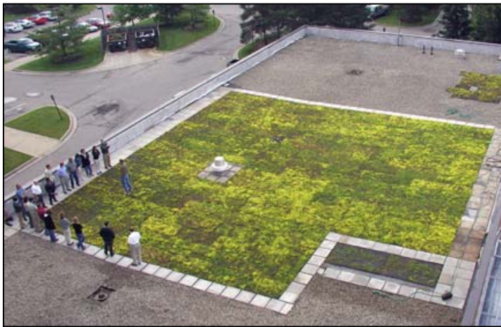
View of the green roof from a fifth floor window of the Plant and Soil Sciences Building
